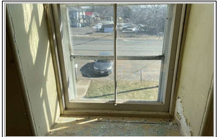
Cracked Window Pane
