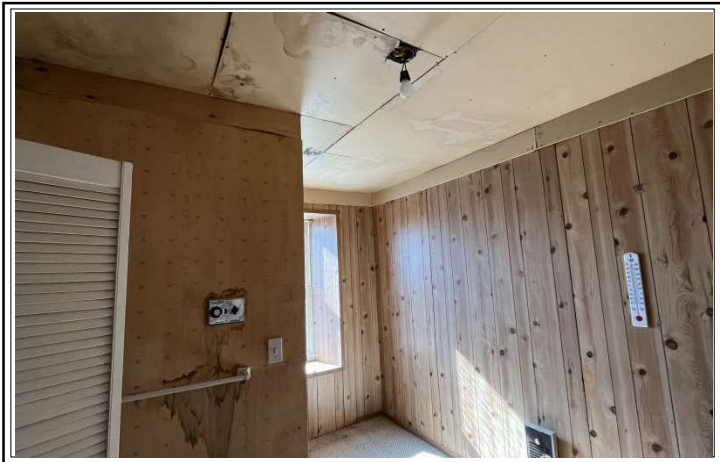
Stained and Damaged Ceiling
